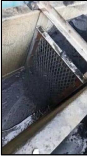
Figure 1: HMV launder grid that has trapped coarse material.
